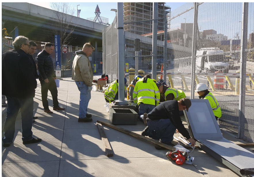
CityEI pilot installation at St. George, Staten Island (NYC Department of Transportation)
