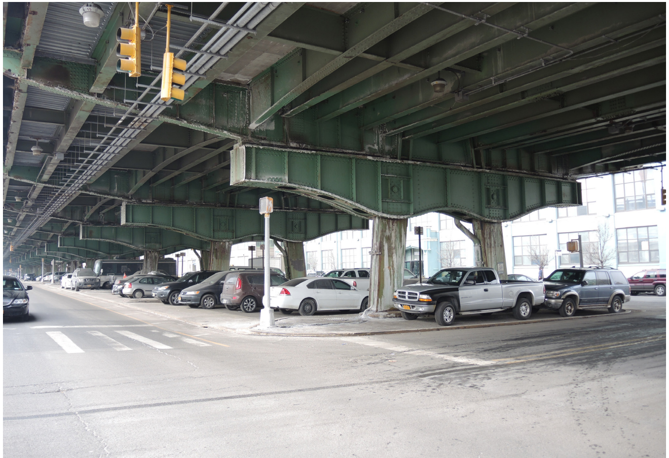
Parking conditions under the Gowanus Expressway at 36th Street and 3rd Avenue before installation of the Sunset Park pilot (Zoë Piccolo)
